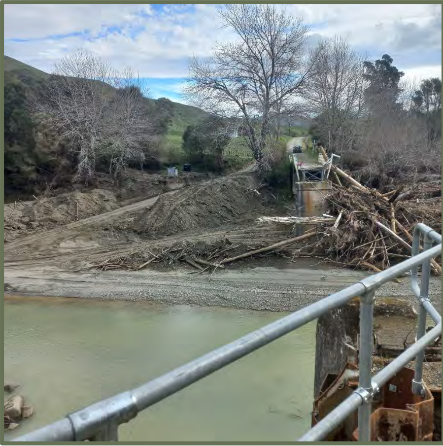
Figure 2-8: Bridge Washed out, east to west view (Civil Assist)
