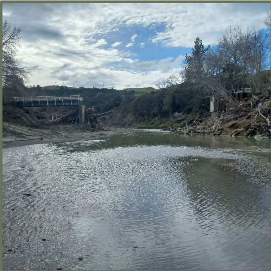
Figure 2-9: Bridge washed out south to north view (Civil Assist).
